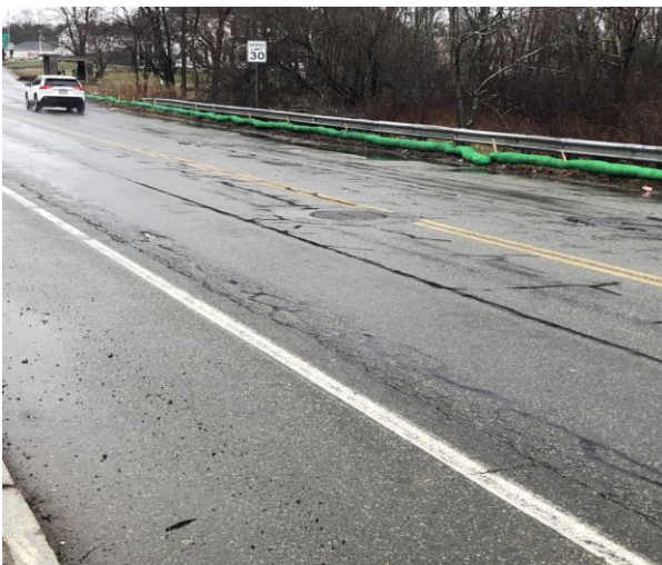
Photo 1: Installed Filter Sock
