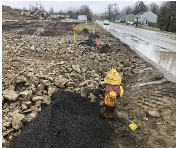
Photo 2: Buried 6" Water Main Bypass Piping
