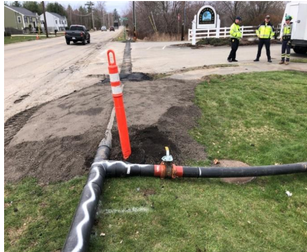
Photo 4: 4" Bypass at Auburnville Way
