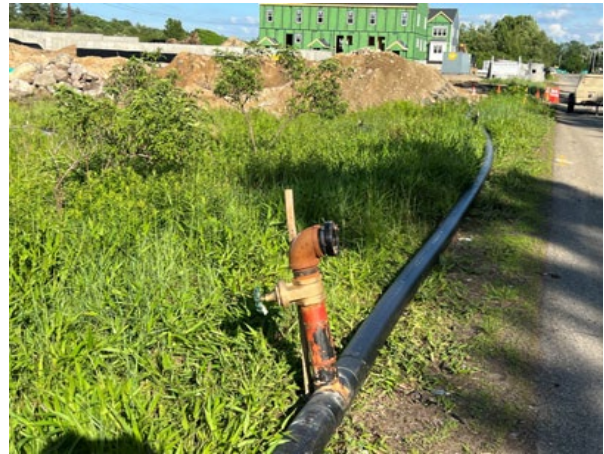
Photo 4: 6" Temporary Bypass Piping Connected to Temporary Hydrant
