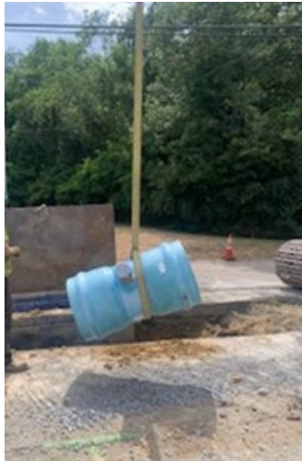
Photo 2: 20-inch x 4-inch Tee on Auburn Street
