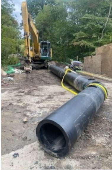
Photo 2: Assembled and Fused 20-inch HDPE Sewer Force Main for Installation in Cross Country Easement
