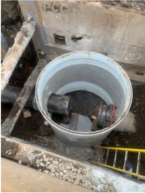
Photo 1: Air Release Valve Manhole in Landfill Easement
